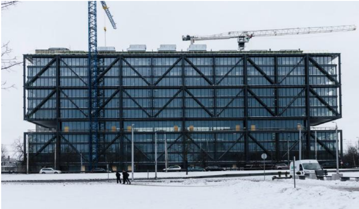
Photo of the Phase A building from the construction site as of January 2026 Source: Issuer
